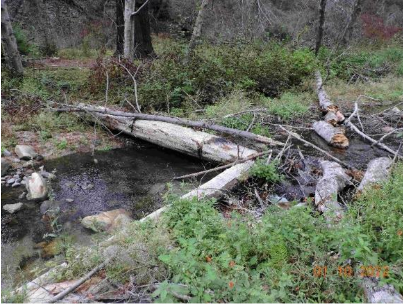
Photo 5. Decades old V-weir was substantially rinsed under the cap logs, mostly eliminating the protected undercut that provided high flow velocity refuge and escape cover. The average depth of the pool below the weir has been reduced by at least half. Streamside alder canopy is mostly gone.
