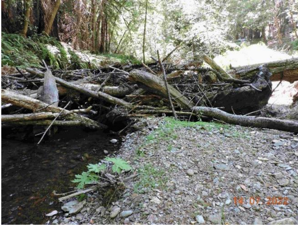
Photo 69. Mile 5.0, just upstream of Slate Creek, viewed from upstream. Large (5 ft high by 30 ft wide) partial wood jam. Presently passable underneath and, at high flows, around the jam on right bank.
